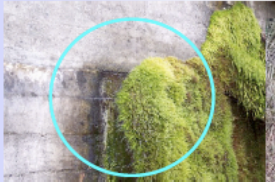
Leaking reservoir wall
