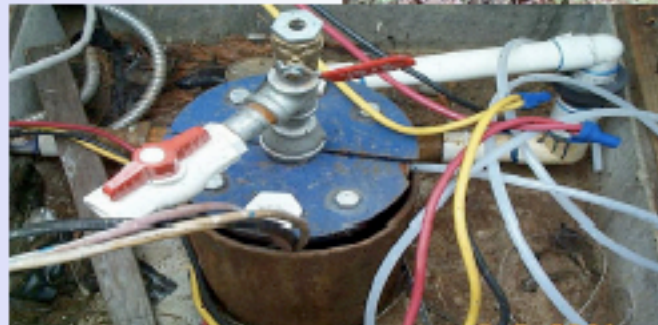
Wellhead that needs to be replaced
