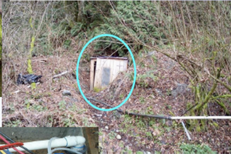
Spring Box with open access
