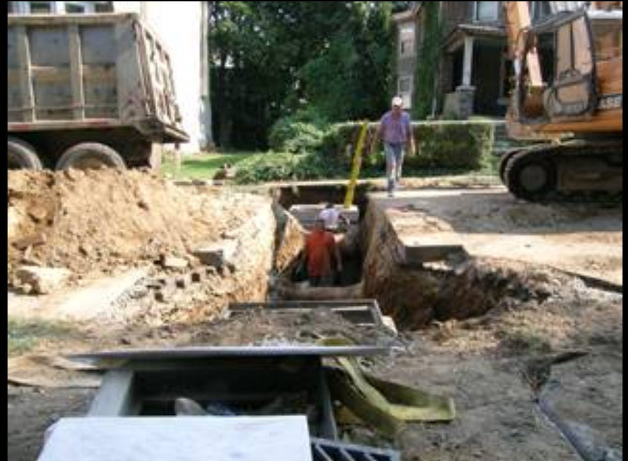
New Inlets to Divert Street Runoff
