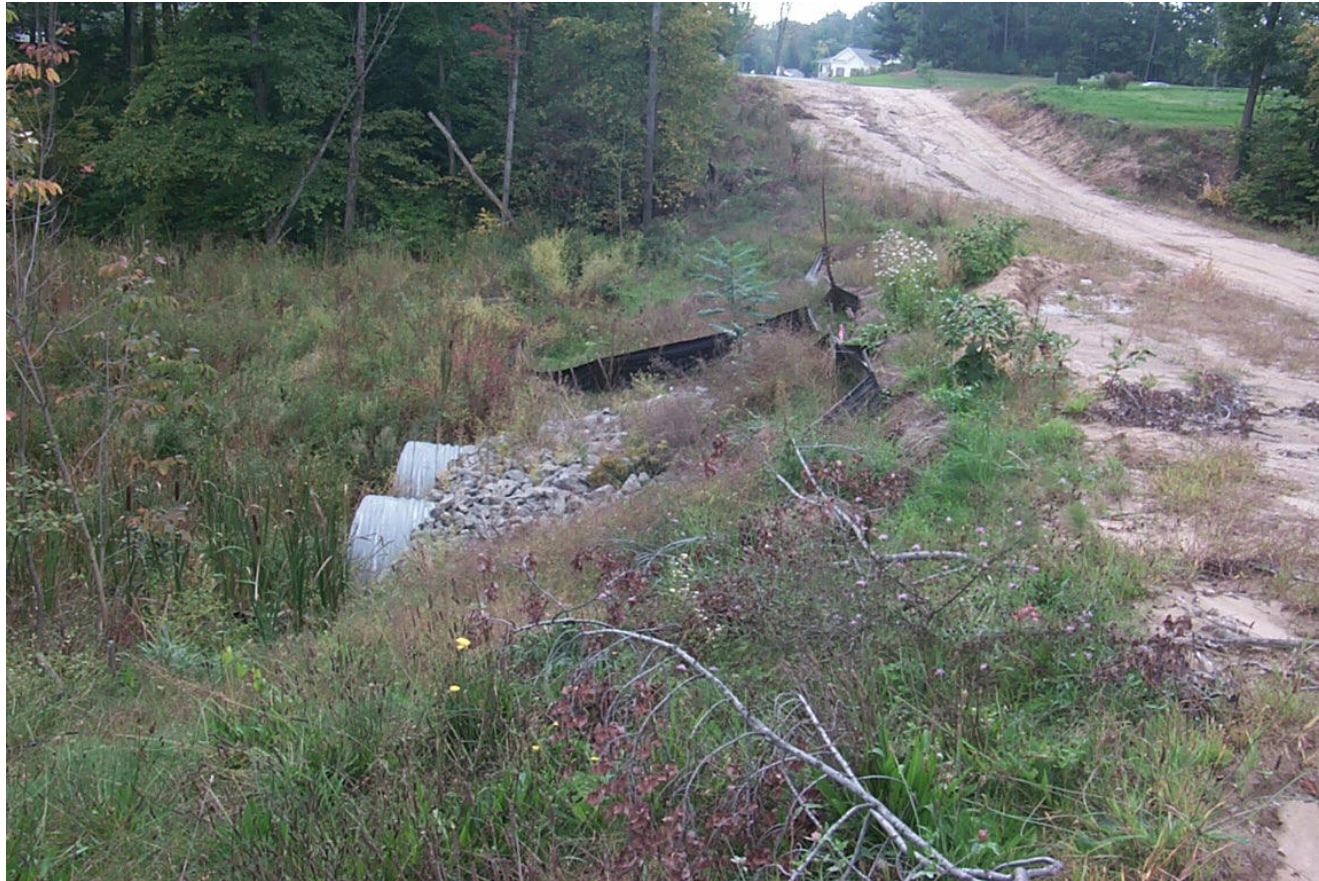
Buried and improperly maintained silt fence adjacent to Normans Kill in new Rotterdam housing development. Proper maintenance of erosion/sedimentation plans is crucial for effective mitigation.
