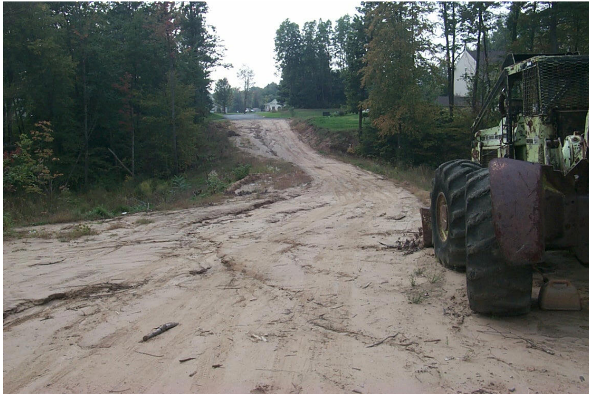
Erosion from housing construction in Rotterdam. At this site, the future road is crossing the Normans Kill.
