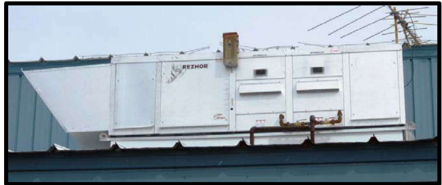
Air Handling Unit, Ice Rink, Saratoga Springs 27
