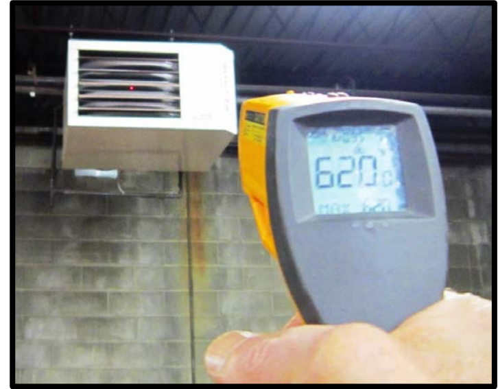
Unit Heater, Clifton Park Garage Why was the temperature so high?
