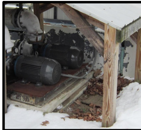
Outdoor Chiller Pumps, Ice Rink, Saratoga Springs
